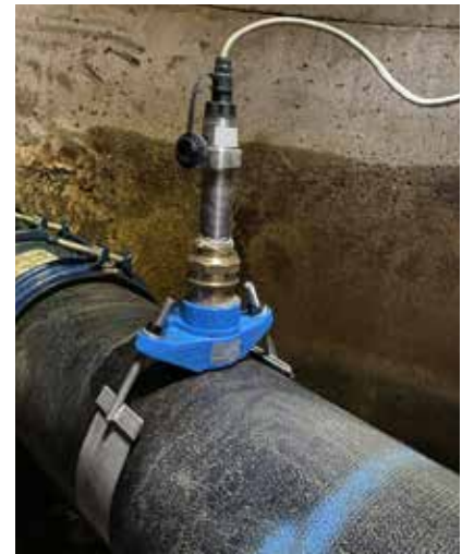
An Aquify flow and pressure sensor on a Buffalo Grove water main.
