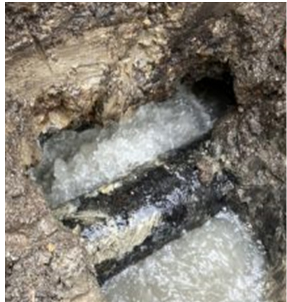
8" cast iron pipe burst identified by Aquify's 24/7 Control Center
